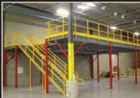
Mezzanine with Elevated Storage
