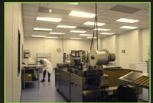
Modular Clean Room
